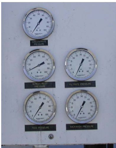
Figure 1b: Example of pressure gauges at different elevations that will need correction.
