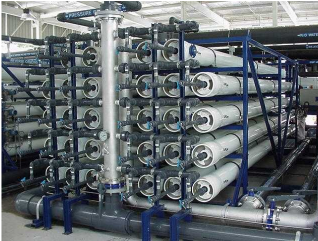
Figure 5 RO Train at Kranji Wastewater Treatment Plant
