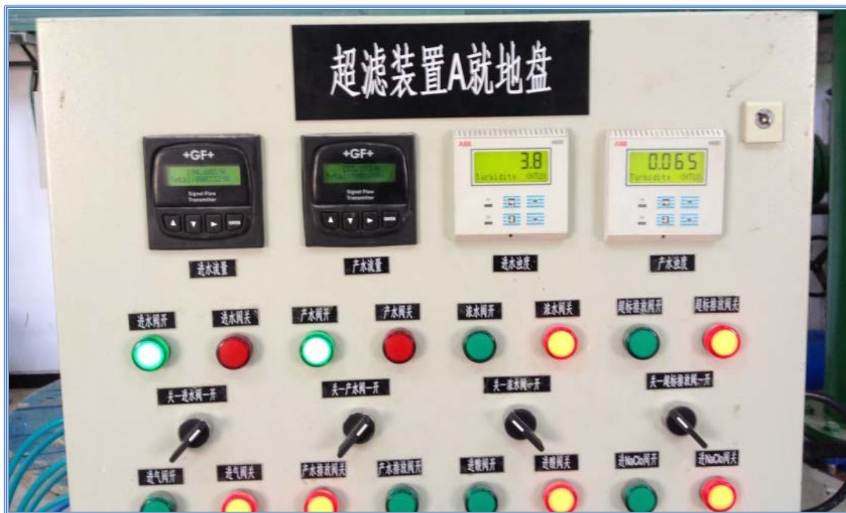
Figure 1: Feed Turbidity (left) and UF Filtrate Turbidity (right)
