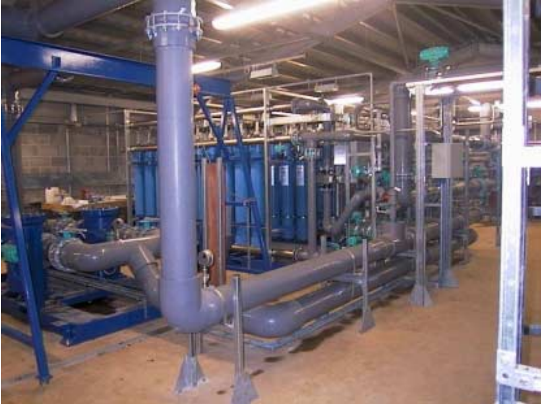
Figure 3 Photograph of the Installation at Frome
