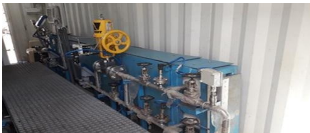
Figure 1. Pilot UHPRO system - 4" dia X 3 element long two vessels in series
