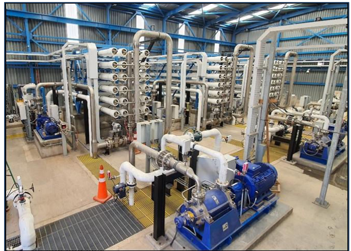
Reverse Osmosis System
