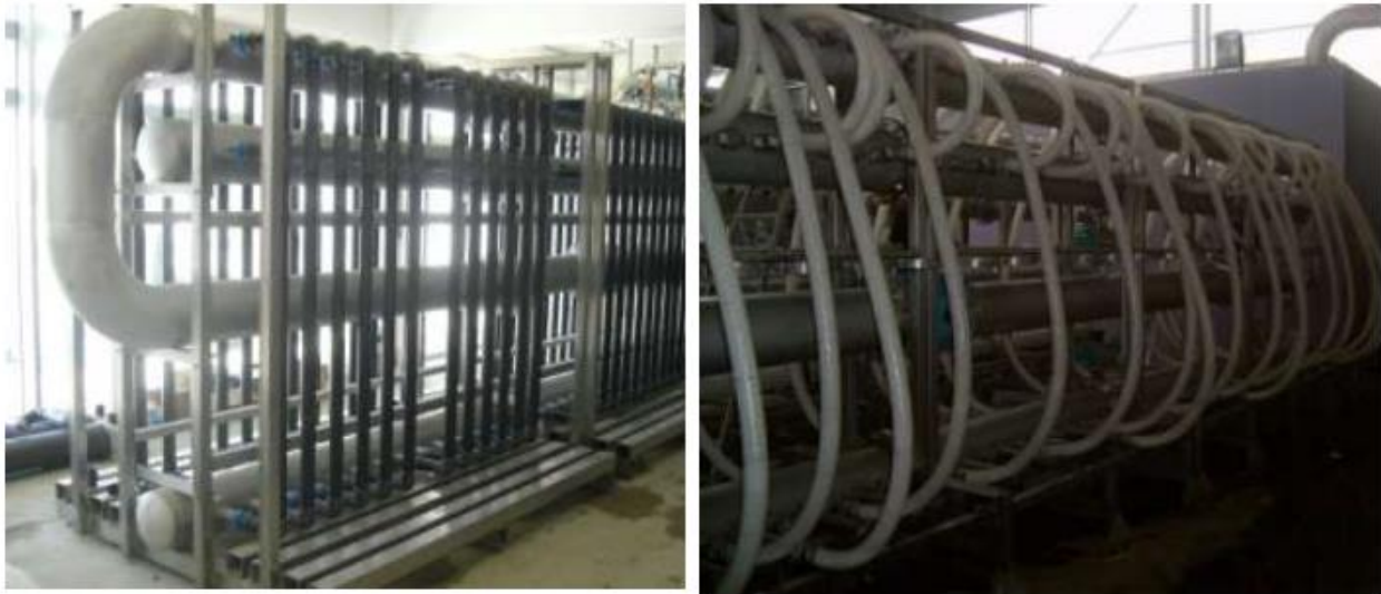
Figure 1: Examples of rigid and flexible piping used for commissioning phase 1.
