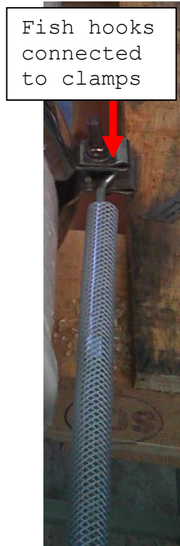
Figure 3: Fish hook connection points on clamps.
