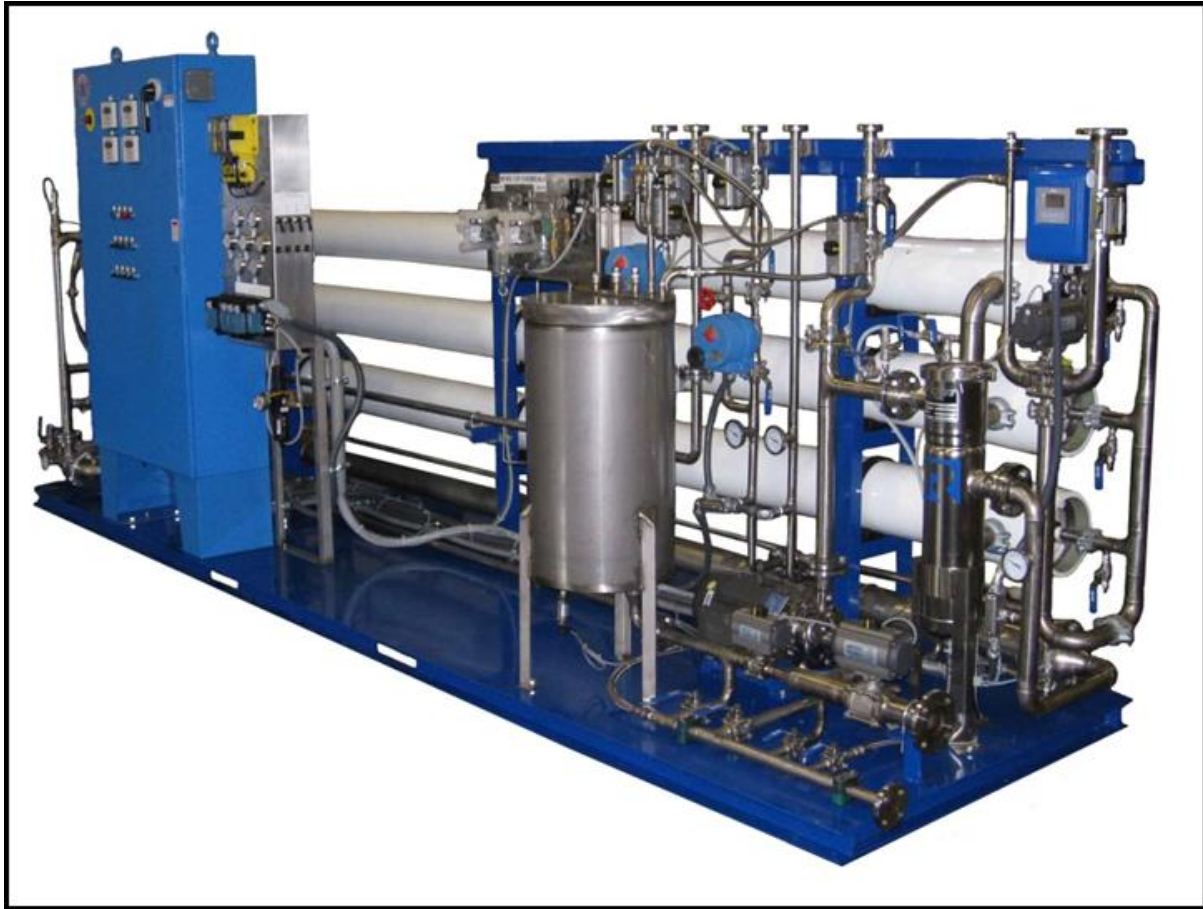
Figure 2: Typical, high temperature RO for laundry waste reclamation
