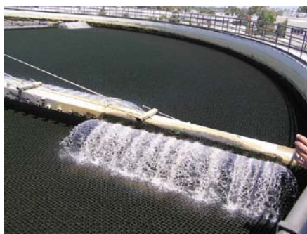
c. Activated Sludge Treatment
