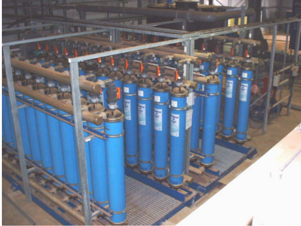
Figure 1: HYDRAcap Installation at Seedy Mill WTW
