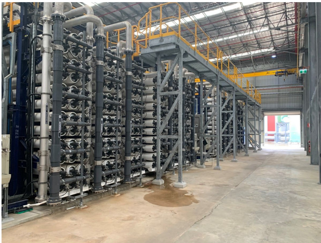
Photo 2 - Beenyup Reverse Osmosis Trains
