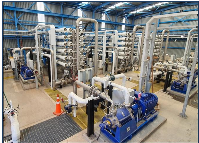
Reverse Osmosis System
